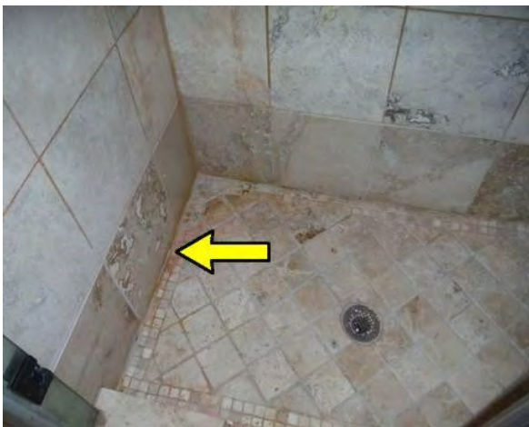
Reseal around base and corners of downstairs shower as required.
