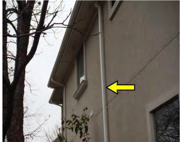
Downspout loose at wall on west side.
