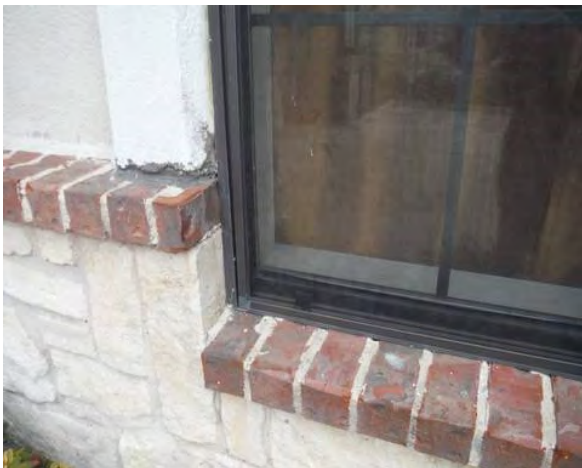
Reseal around windows as required.
