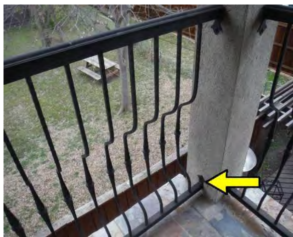
West railing loose at north balcony.
