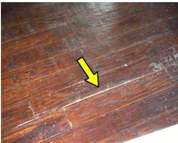
Wood buckling in family room.
