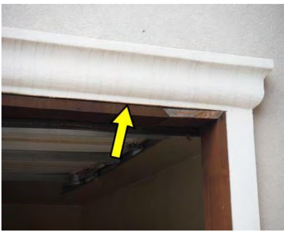
Reseal around garage door trim.
