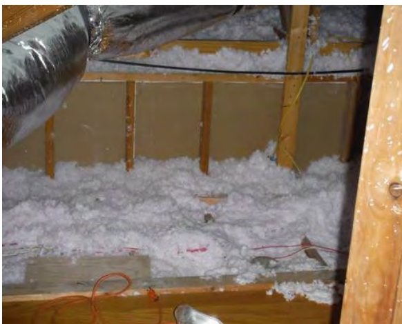
Missing batting insulation on south attic wall of media room.
