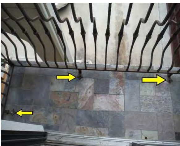
Missing fasteners at the balcony railing feet.
