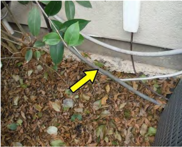
Insulation missing on refrigerant line.
