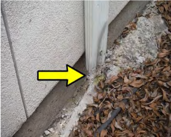
Downspout leader missing on west downspout.
