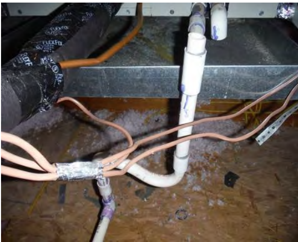
Vent is installed on incorrect side of p-trap on north unit. Cap existing vent and install new vent.
