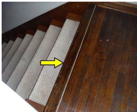
Top tread at landing is loose.
